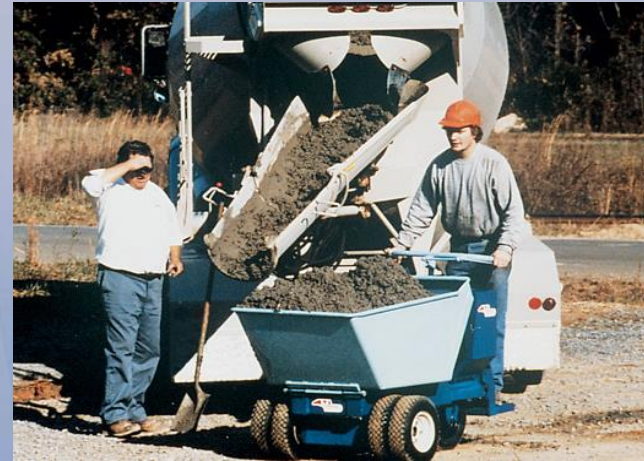
Truck Mounted Conveyors
