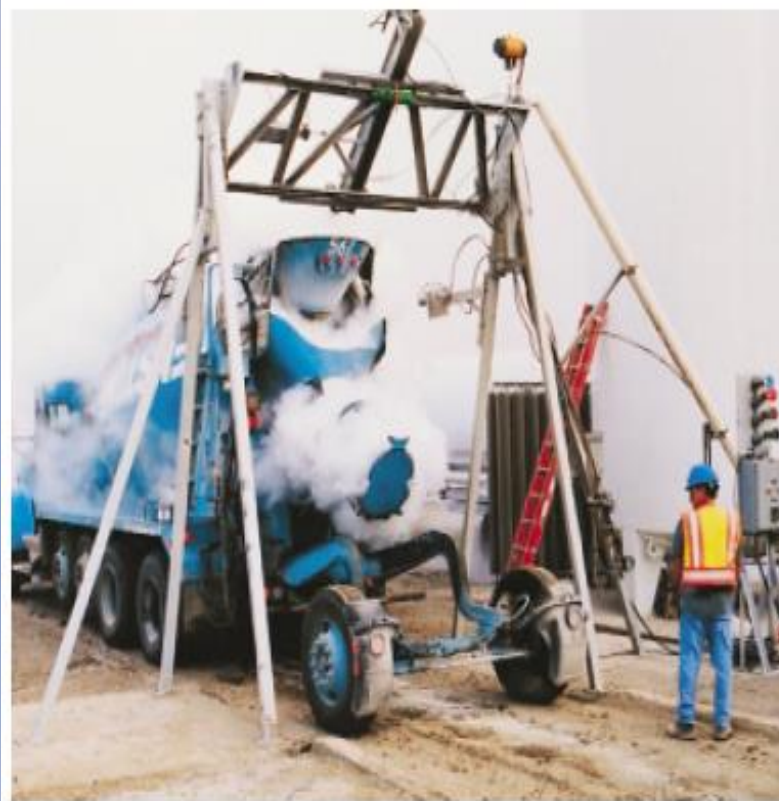
Fig. 13-1. Liquid nitrogen added directly into a truck mixer is an effective method of reducing concrete temperature for delivery to mass concrete placements or during hot-weather concreting. (IMG12357)
