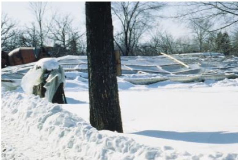
Fig. 14-17. Even in the winter, an outdoor swimming pool can be constructed if a heated enclosure is used. (IMG12269)
