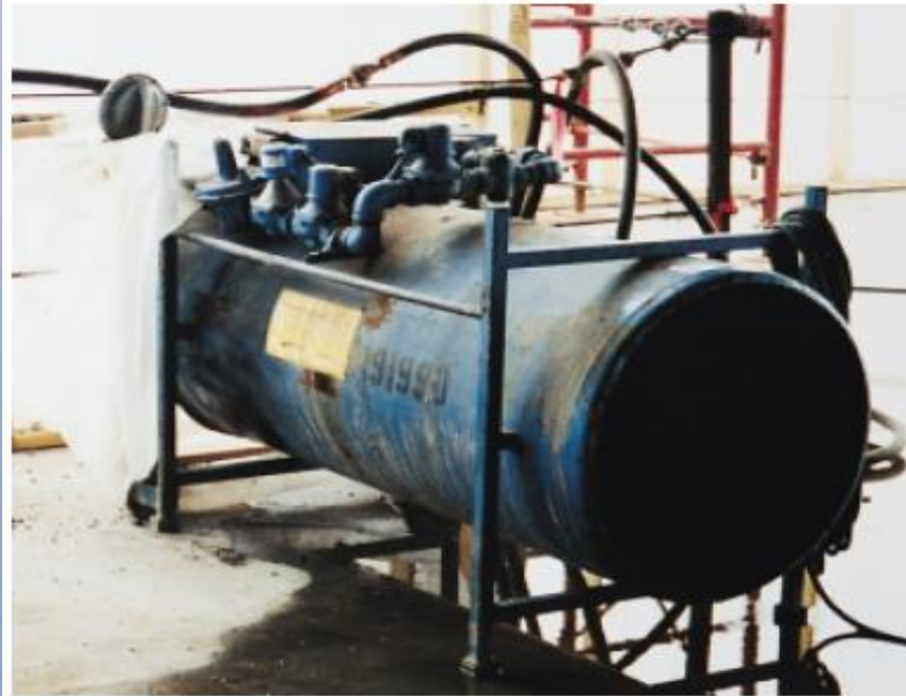
Fig. 14-24. A direct-fired heater installed through the enclosure, thus using a fresh air supply. (IMG12206)
